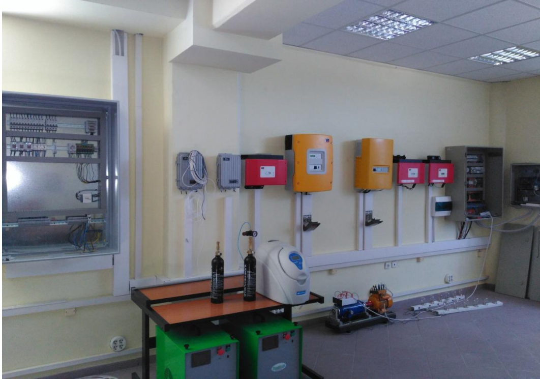
Fig. 7: The two microgrids, as they are installed today at the new facilities.
